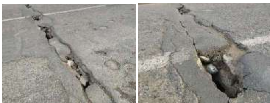
Fig. 3. Defects and damages caused by deformation seams
