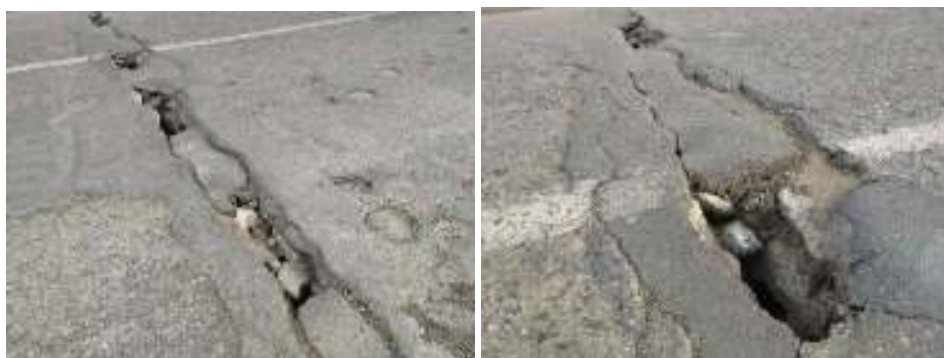
Fig. 3. Defects and damages caused by deformation seams
